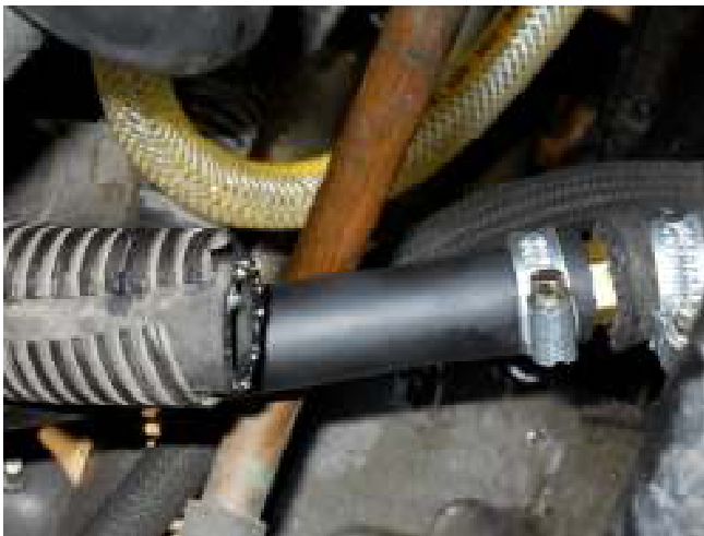
This picture is of the coolant line coming off the engine that was cut. The right side has been connected to one of the installed coolant lines, and the left side is still open. It will be connected to the other coolant line
